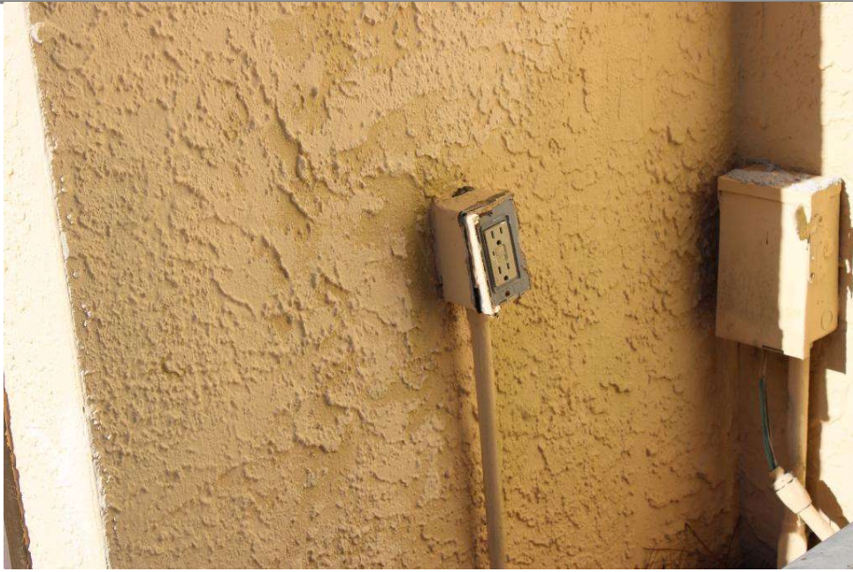
Electrical-Annual Routing Maintenance
