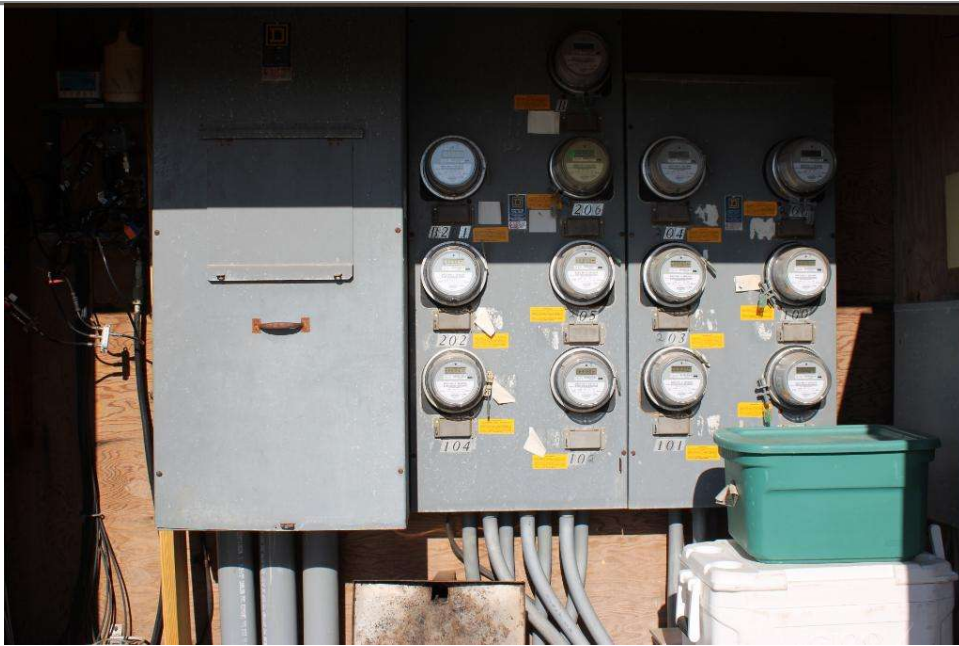
Electrical-Annual Routing Maintenance
